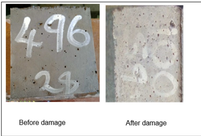
Figure 7: The extent of surface deterioration became evident after exposure to varying wet-dry cycles in the concentrated biogenic sulfuric acid
